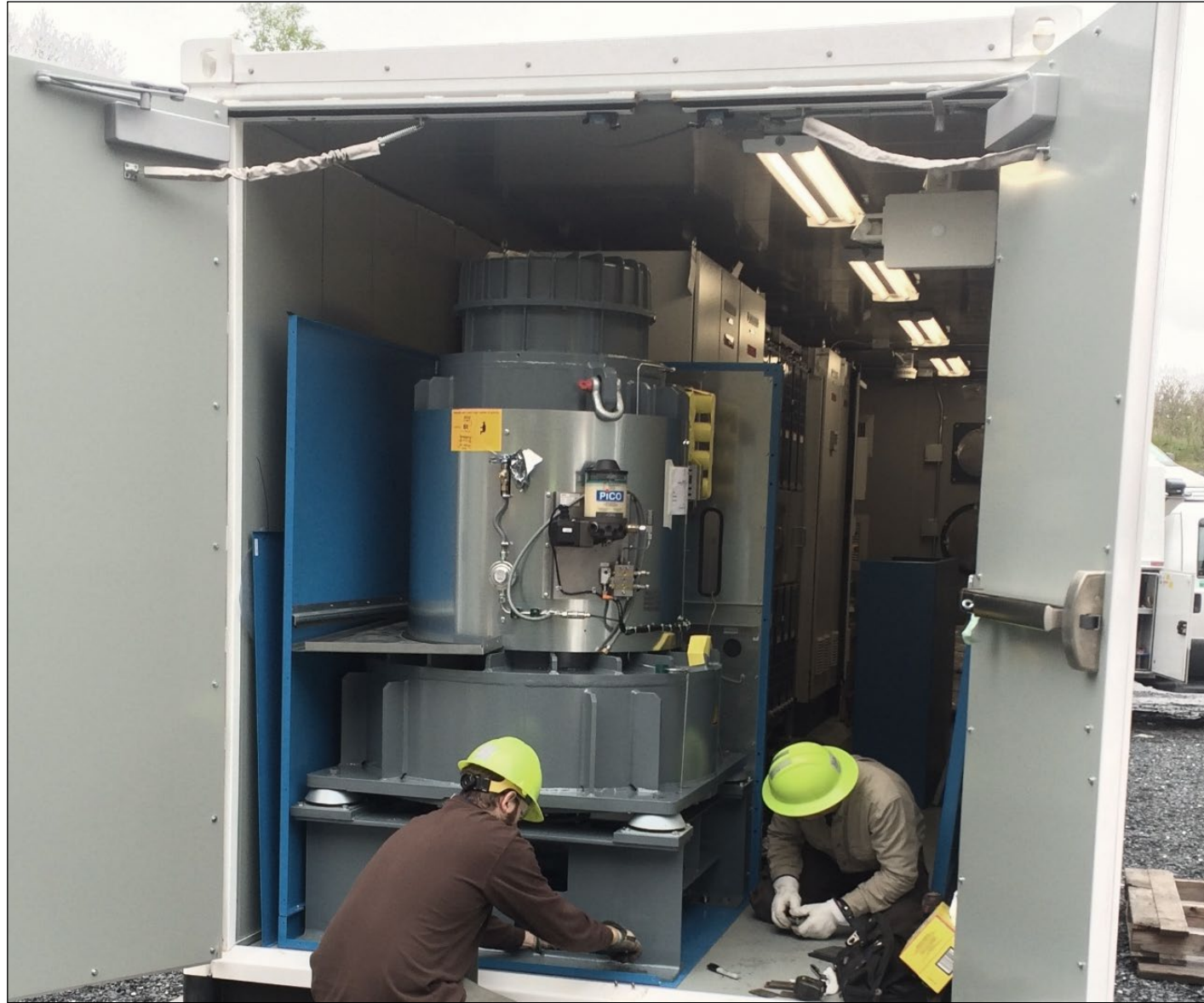
Flywheel Energy Storage System
