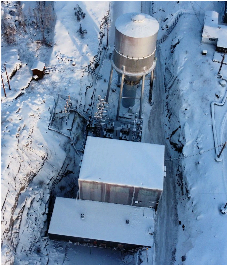
Taltson Hydro Facility
